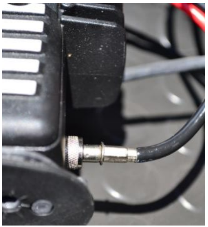
Coax cable into the back of your radio (in trunk) should be hand-tight.
